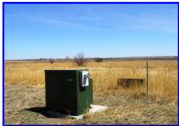
Heavy Electrical Transformer on property
