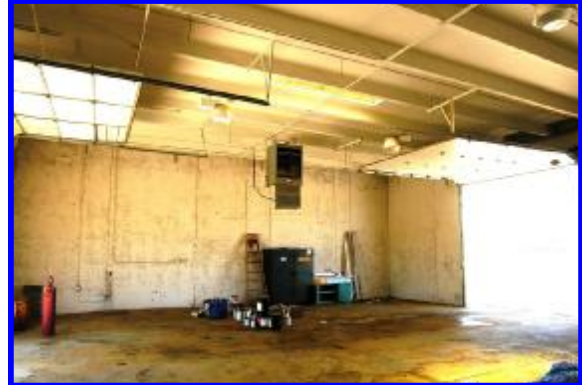
South Side Interior—Propane Space Heater
